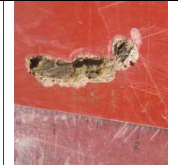
Figure 3: Larger diameter fault showing deeper pitting.
