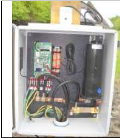
Figure 4: AC mitigation facility with monitor system.
