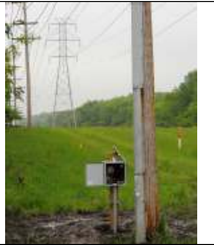
Figure 5: Mitigation facility installed on right of way.
